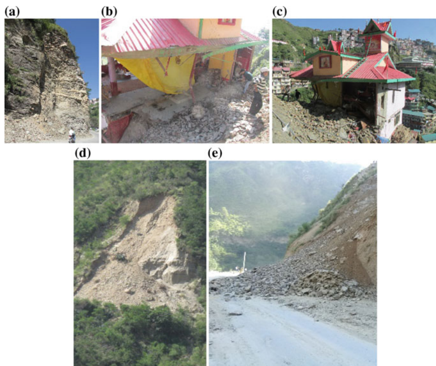
Fig. 9 a Rock slide occurred along the NH 5A in Shimla town. b and c settlements damaged due to the landslide. d and e landslide occurred along a place called Luhri located in Shimla—Rampur National Highway
