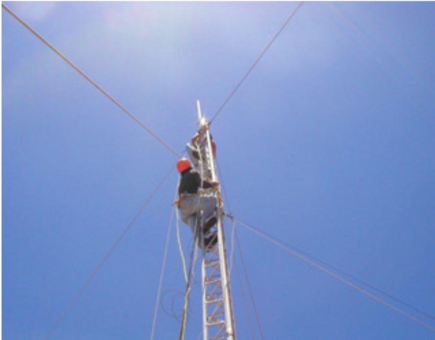
Figure 8.2: A climbable guyed tower.
