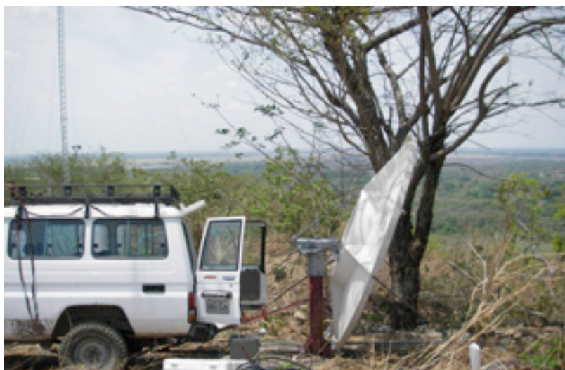
Figure 11.34: El Baúl antenna installation. Actual elevation was 1^\circ upward, since the antenna has an offset of 22.5^\circ .
