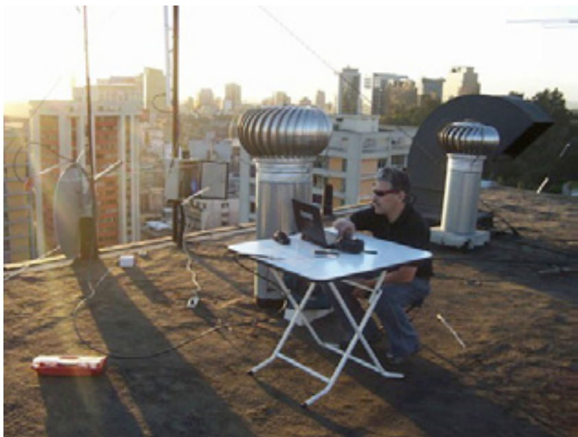
Figure 11.23: Downtown node connected to the Santiago southern node. Note the parabolic antenna for backhaul and the slotted antenna to connect the clients.
