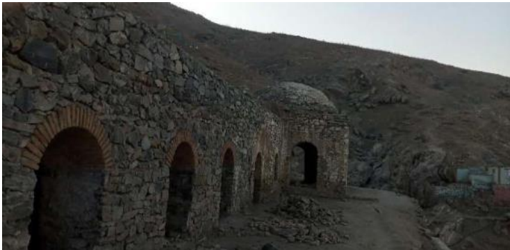
Front elevation Pictures of the Buddhist temple after renovation from the east
