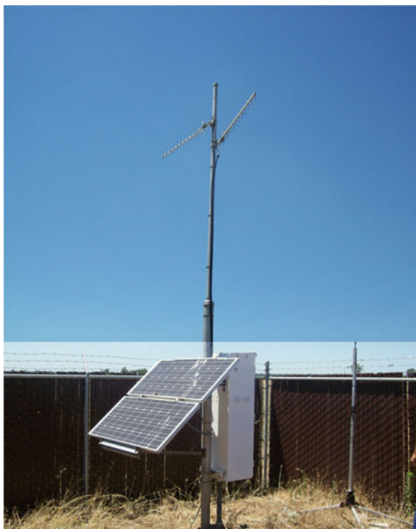
Fig. 6.3 GNSS CORS power supply and telemetry
