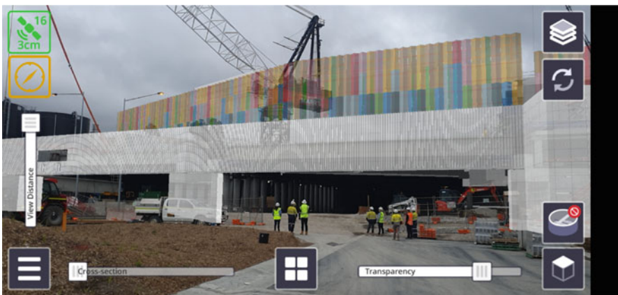
Fig. 1.7 A snapshot of SiteVision AR in real-time overlay of design data of the tunnel facade onto the existing conditions at the work location in The M4-M5 Link Tunnels project in Sydney, Australia, in 2021. Image used by permission. Courtesy of WestConnex ( westconnex.com.au )
