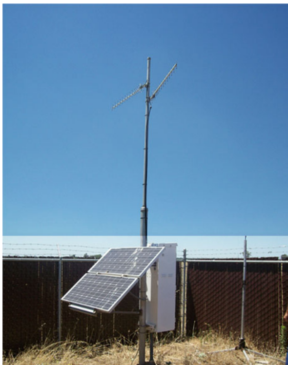
Fig. 6.3 GNSS CORS power supply and telemetry
