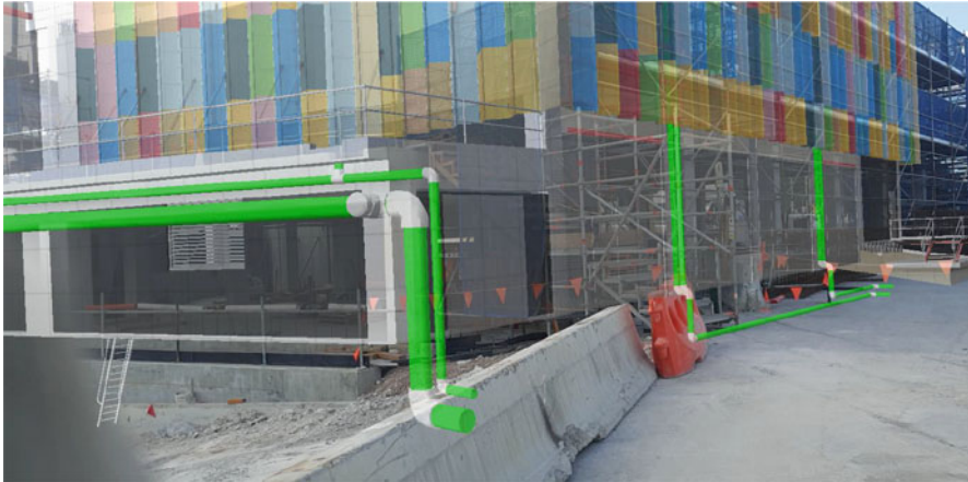
Fig. 1.6 A snapshot of SiteVision AR in real-time overlay of the design data of pipes and conduits onto the existing conditions at the work location in The M4-M5 Link Tunnels project in Sydney, Australia, in 2021. Image used by permission. Courtesy of WestConnex ( westconnex.com.au )
