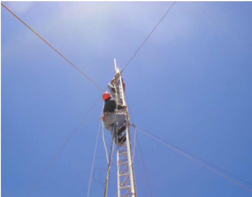
Figure 8.2: A climbable guyed tower.
