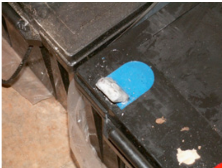
Figure 7.2: A 200 Ah lead-acid battery. The negative terminal was broken due to weight on the terminals during transportation.
