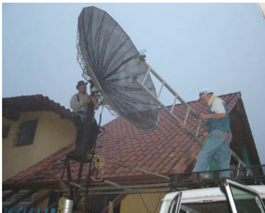
Figure 11.30: Carlo and Ermanno disassembling the satellite dish supplied by Mr. Ismael Santos.
