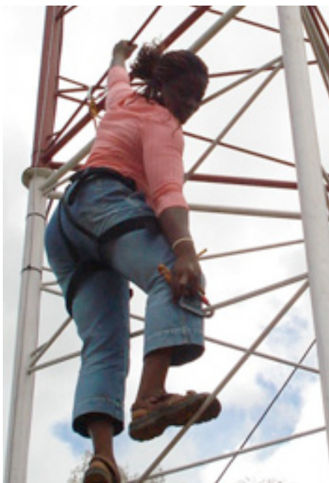
Figure 11.3: Omolayo Samuel, one of the staff of Zittnet, does not fear the height of the 45m tall tower as she is aligning the antennas hosted in the top of the tower.
